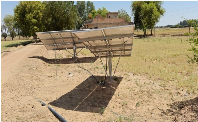
Fig. 3: Solar-powered pump installation on a farm
