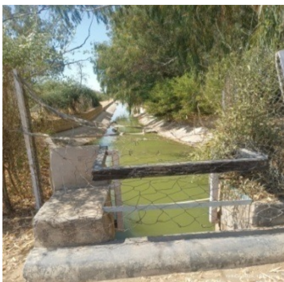
Fig. 1: Canal outlet structure in the arid zone
